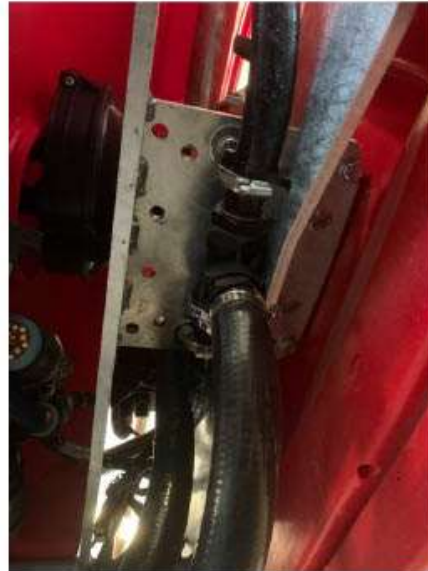
Figure 5: Pressure side T piece, under the fan bearing block
