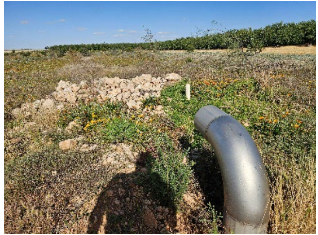
Purge Valve Outlet
