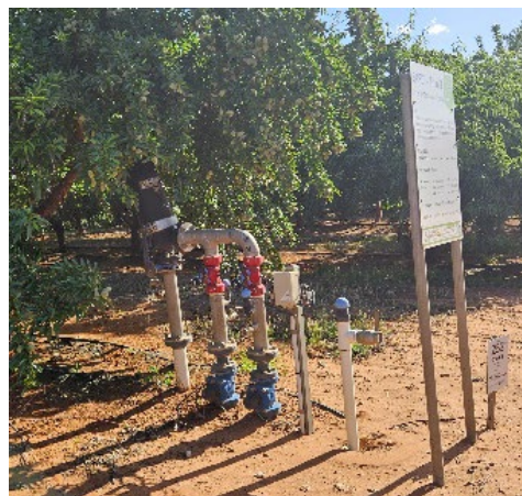
Twin Valve Manifold and Laterals
