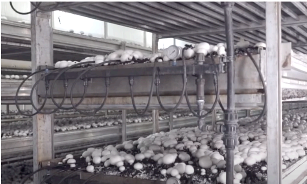
Figure 56. Netafim "Mushroom Master" irrigation system
