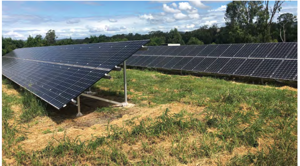
Sandbar Citrus started investing in solar about 11 years ago, but in the past two years their solar installations have increased in size and they are reaping the benefits for lower cost electricity.
